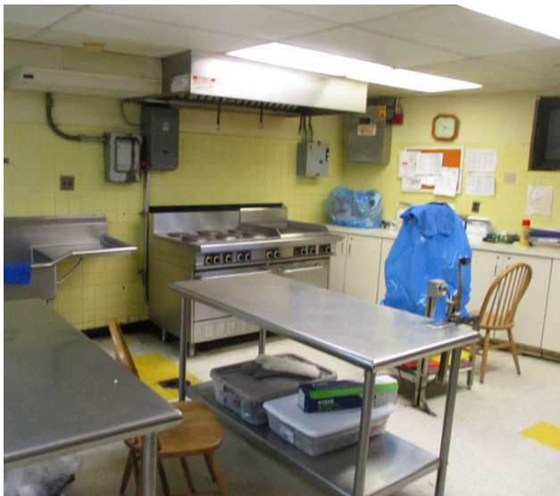
Kitchen appliances and finishes
