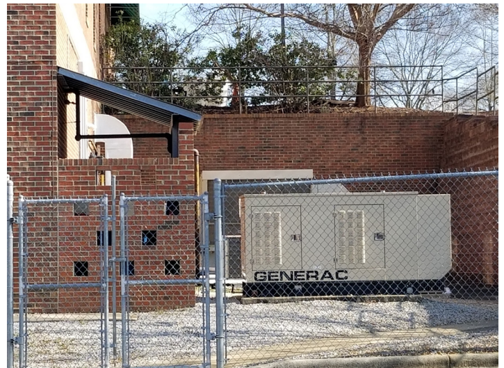
300 amp Generator Serves as Back-up Power - Natural Gas Fired
