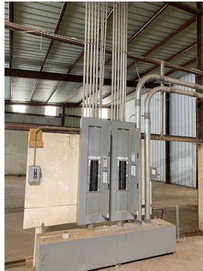
400 amp, 3-phase power
