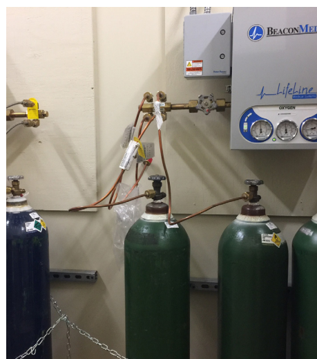
Gas Tank Closet
