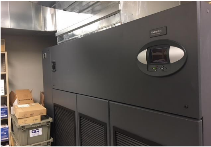
LIEBERT HVAC 12.5 TON COLLING SYSTEMS
