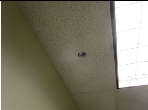
Photo 31: View of fire sprinkler head (typical)
