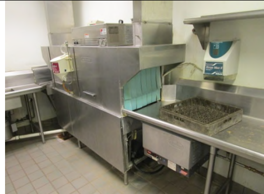
Photo 46: View of automated dishwasher on ground floor
