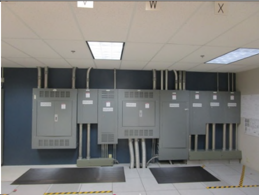
Photo 41: View of electrical subpanels in data room
