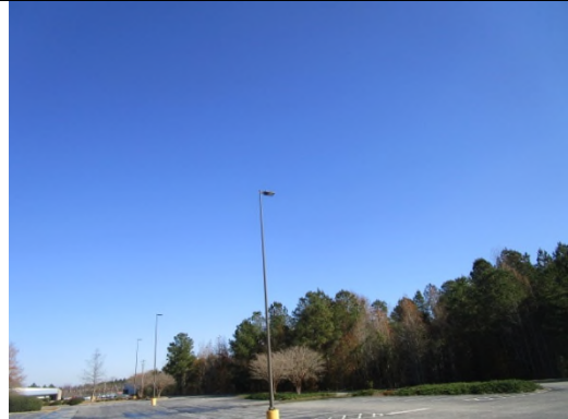
Photo 6: View of site lighting in east parking lot (typical)
