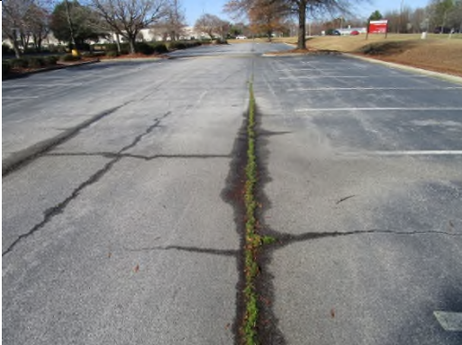
Photo 11: View of vegetation in asphalt cracks in west parking lot
