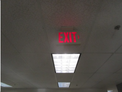
Photo 33: View of lit egress signage (typical)
