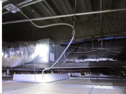
Photo 26: View of above ceiling air handling unit and ducts (typical)
