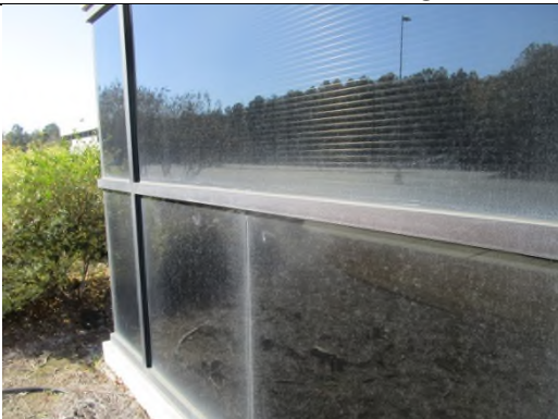
Photo 55: View of acid rain staining on ground floor windows at northeast corner of building
