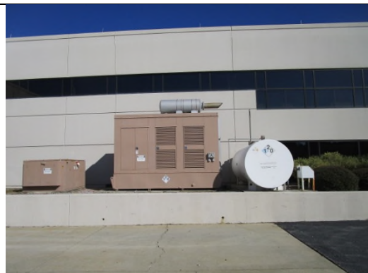
Photo 16: View of emergency backup generator at east loading dock area
