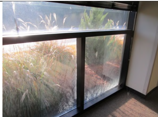
Photo 54: View of acid rain staining on ground floor windows at northeast corner of building
