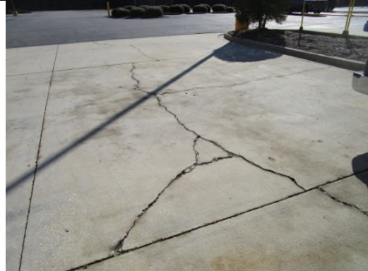
Photo 12: View of cracks in concrete loading dock pavements
