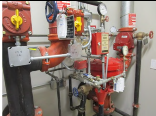
Photo 30: View of fire protection sprinkler system
