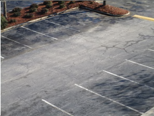
Photo 9: View of cracks in parking lot asphalt pavements (typical)
