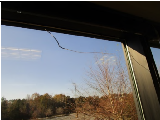
Photo 53: View of cracked window on south end of second floor of building
