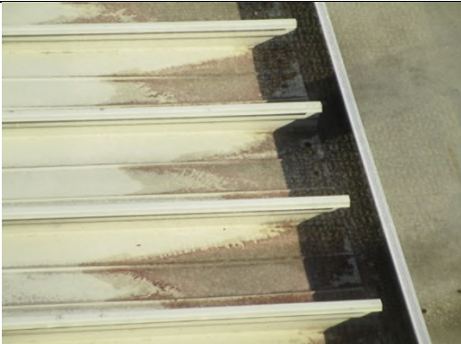
Photo 23: View of rusted metal roofing over patio on east side of building
