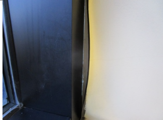
Photo 38: View of peeling wallpaper in north office area on ground floor
