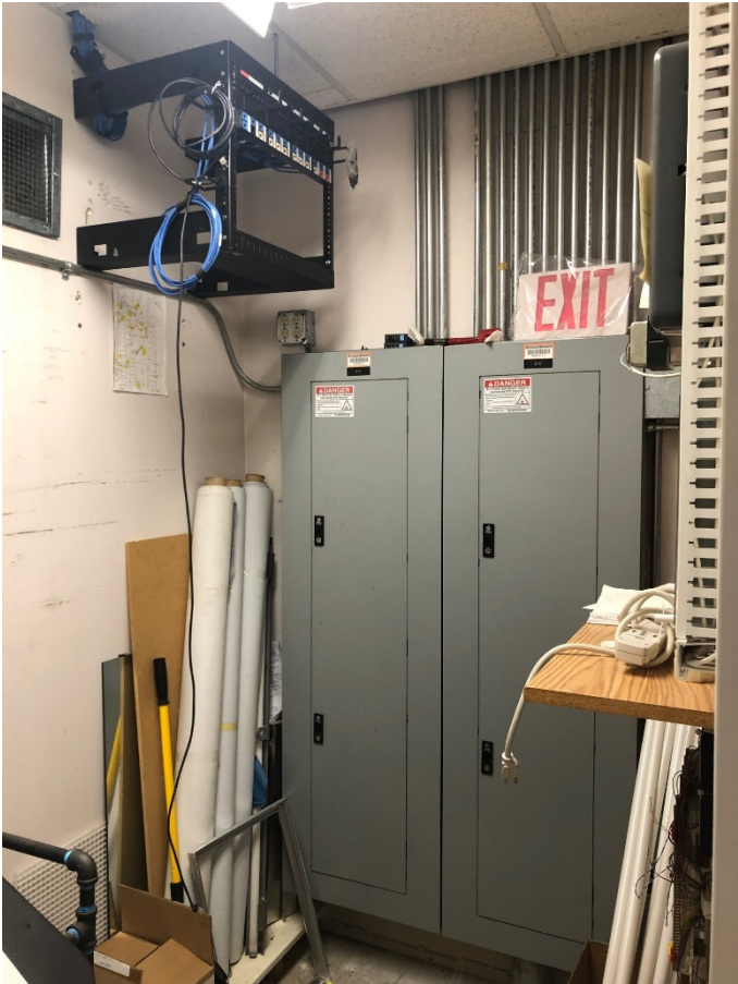
ELECTRICAL PANELS/UTILITY ROOM
