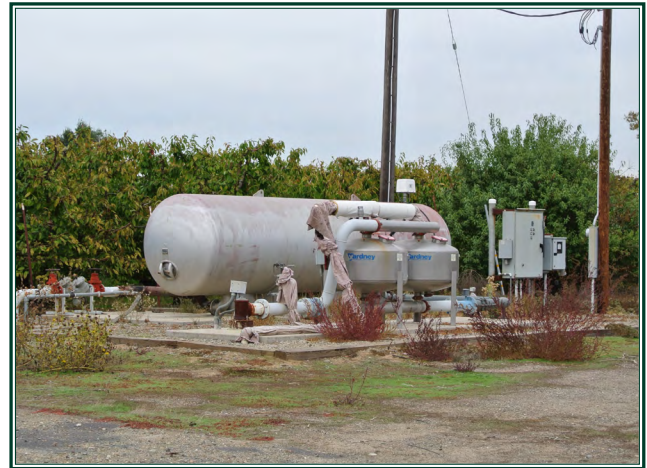
500± foot well with 50 HP submersible pump.
