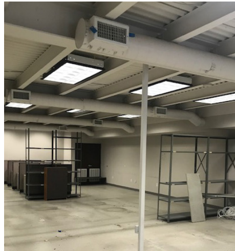
Work area with HVAC
