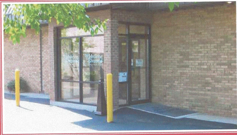
Newly added/constructed side entrance for more convenient access to rear parking lot.
