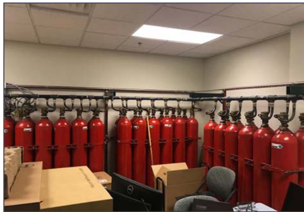
Data center fire protection
