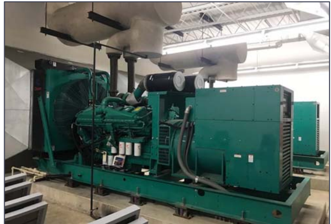
1 of 2 Onan generators
