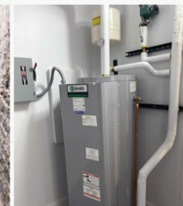
BRAND NEW WATER HEATER
