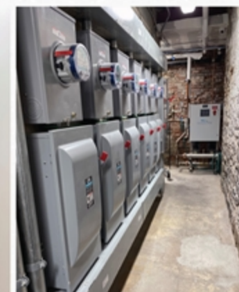
BRAND NEW METER ROOM
