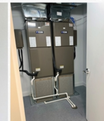
BRAND NEW HVAC EQUIPMENT
