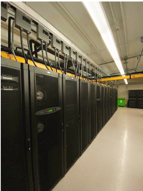
Existing data center
