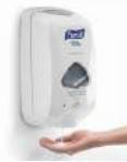
WALL MOUNTED TOUCH-FREE PURELL HAND SANITIZER AT ENTRANCE TO PANTRY GRAB & GO AREAS AND COPY AREAS
