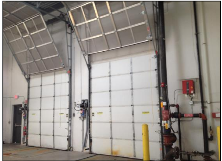
Dock Doors with Screens and Truck Locks (10'x12')
