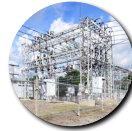
ON-SITE POWER PLANT
