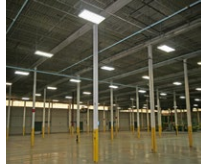
NEW T-8 LIGHTING
