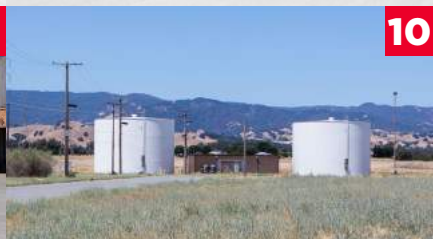
Water Tanks and Sprinkler Pumps
