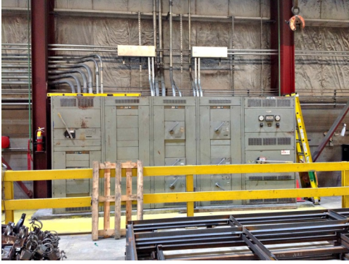
1500 KVA Power, 480 Volts, 16,000 Amps
