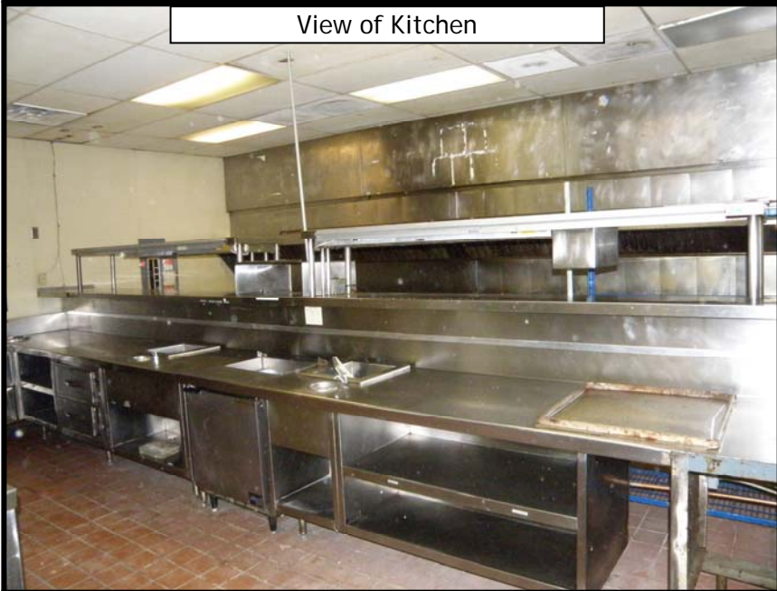
View of Grills/Exhaust System
