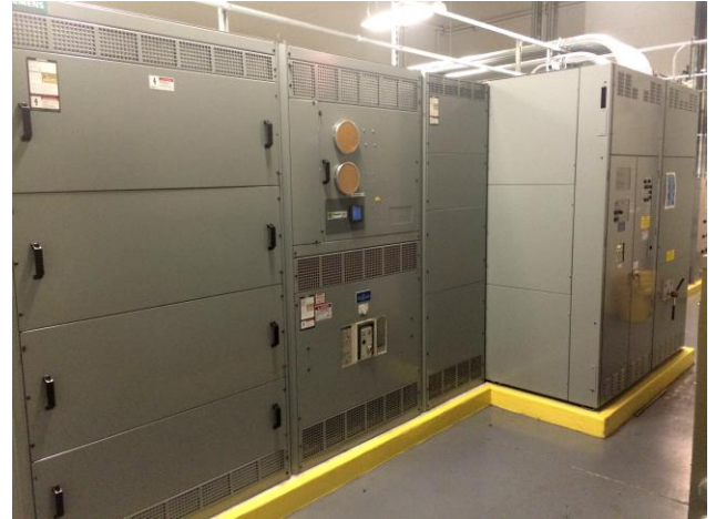
\pm 7,500 kVA Electrical Capacity
