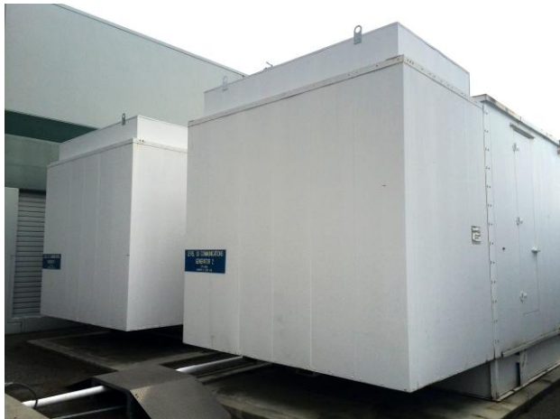
3 \pm 2,000 kW / \pm 2,500 kVA standby diesel generators
