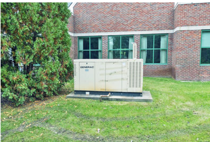
Hard-wired Gas Generator
