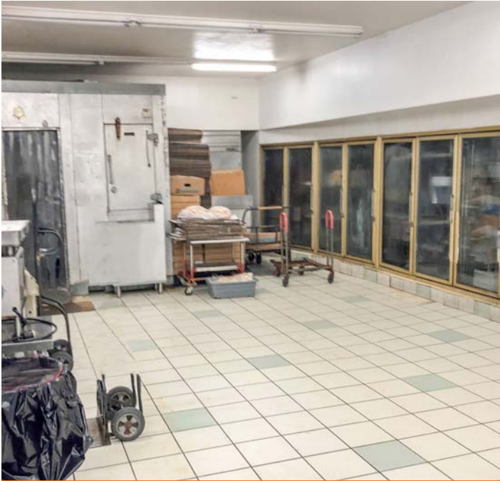
Walk-in coolers and freezer
