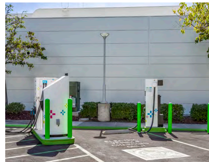
EV CHARGING STATIONS
