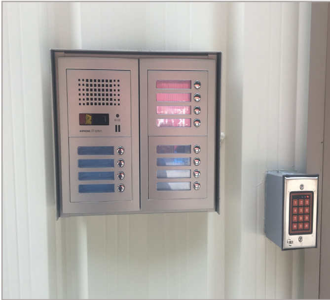
New keypad entry system
