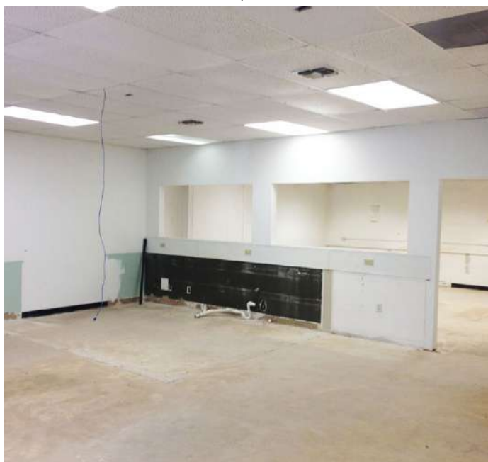
Water & Sewer are located in the half wall of Workshop Area #2.
